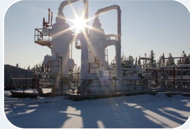
Gas treatment unit No.102 at Kovyktinskoye field
